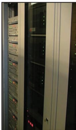
Darlex units with expansion boxes in the Havering control room
