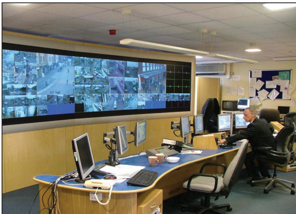
The modern control room at Havering Borough Council
